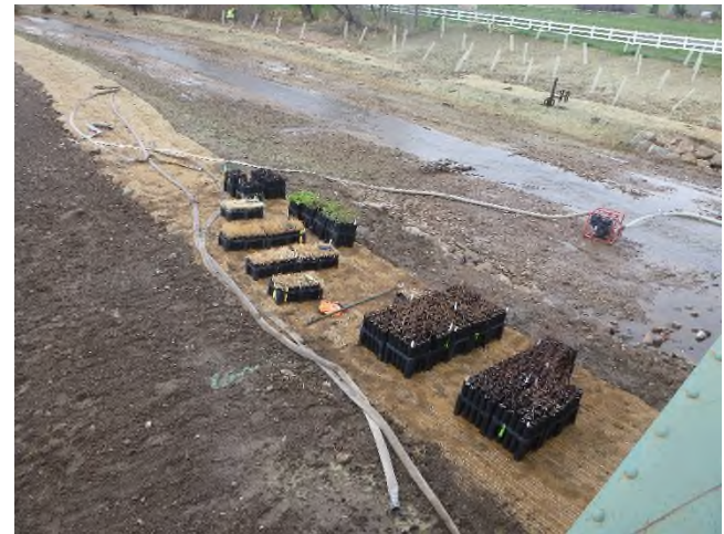
Figure 2 – Container plants on the right bank, upstream of the bridge, waiting to be installed.
