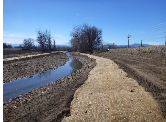
Figure 1 – Looking upstream near Sta 3+00. The river has been returned into the main channel and the diversion ditch has been covered over. Willows and erosion control blanket visible.
