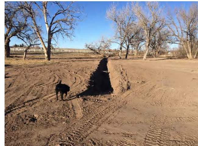
Figure 2 – Looking north near Station 22+00 at the newly created Elgin ditch. The ditch will not connect to the main channel under this project.
