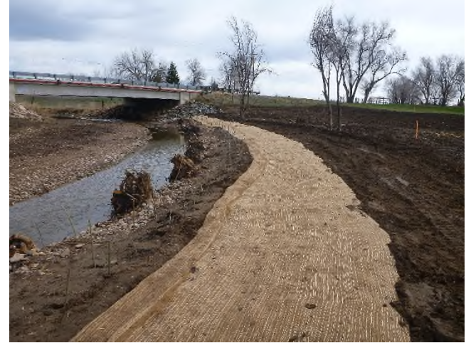
Figure 1 – Looking downstream near Sta 1+00 at the newly installed willows and erosion control blanket on the right bank.
