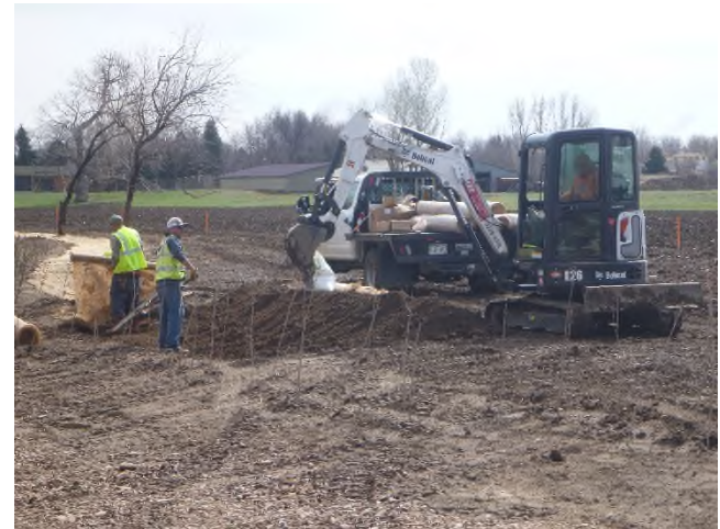
Figure 2 – Look South near Sta 10+50 at erosion control blanket being installed on the right bank. Willows are already in place.
