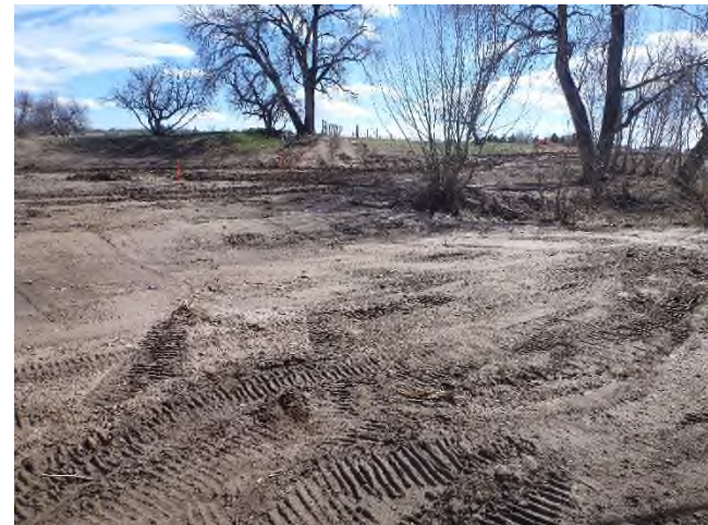
Figure 2 – Look South near Sta 11+50 at the swale graded into the floodplain to allow the wetlands to drain any standing water.
