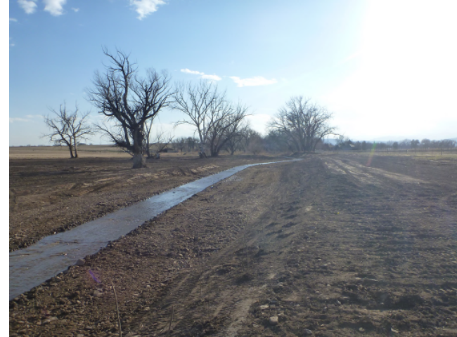
Figure 1 – Looking upstream near Station 24+00 at the recently graded channel and floodplain. Willows are visible in the foreground.
