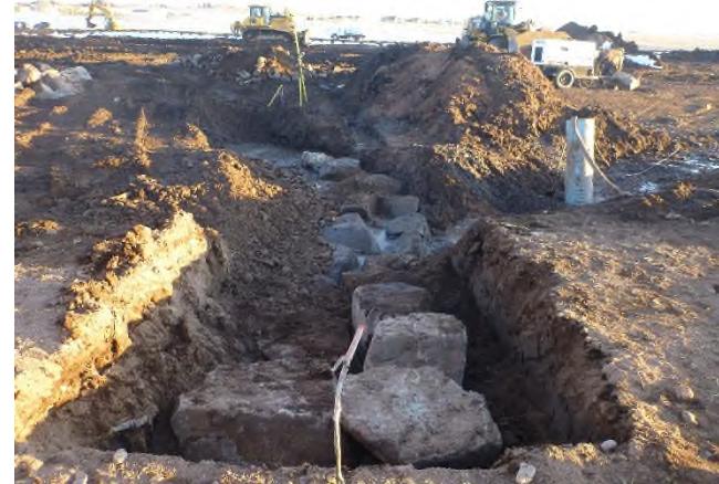
Figure 1 – Looking South across the channel at approximately Sta 22+50 at the at-grade boulder structure under construction.
