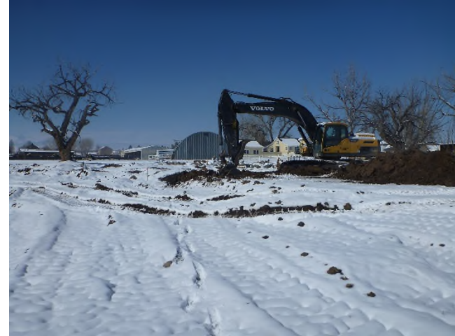
Figure 1 – Looking upstream near Station 21+00 at rootwads being installed on the left bank (photo right).
