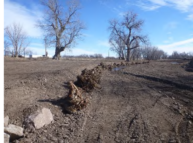
Figure 1 – Looking downstream near Sta 15+00 at the final channel shaping with design bed material. Completed rootwads are visible at left.
