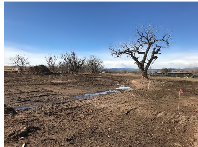
Figure 2 – Looking upstream near Sta 21+00 at the coarse channel grading. Channel bed material and final channel shaping has not yet occurred. Ground water seepage visible.
