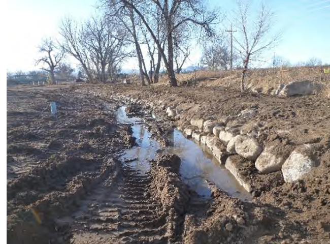
Figure 1 – Looking upstream at the newly completed stacked boulder bank at Sta 10+00. The channel will be constructed out of the design bed material up to the top face of the toe boulders.
