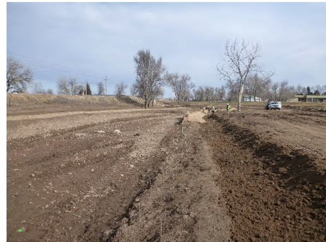
Figure 2 – Looking downstream near Sta 4+50 at the erosion control blanket and willows being installed. A boulder cluster is visible on the head of the point bar near the low flow channel.
