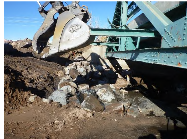
Figure 2 – Stacked boulder wall being constructed around the Green Bridge. (Photo taken from the upstream side of the bridge looking north.)
