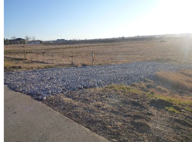
Figure 1 – Looking south at newly installed vehicle tracking pad on the upstream side of the Green Bridge. Mountain River Road is at photo left in the foreground.
