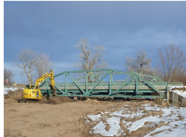
Figure 2 – Looking downstream at the upstream face of the Green Bridge. Material is being removed from underneath the bridge. The ground is partially covered by ice and snow.
