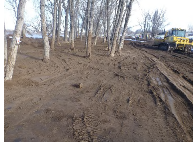
Figure 1 – Looking downstream near Sta 7+00 at the floodplain grading in the gallery zone on the left bank. Coarse channel grading is underway at right.
