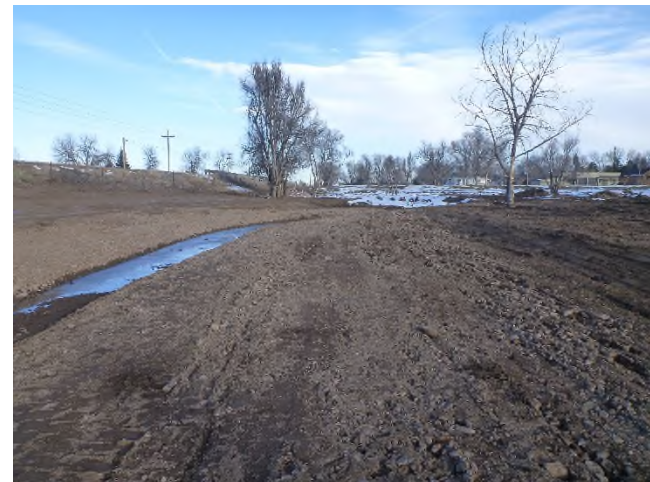
Figure 2 – Looking downstream at fine channel grading near Sta 4+00. Design channel bed material has been placed.
