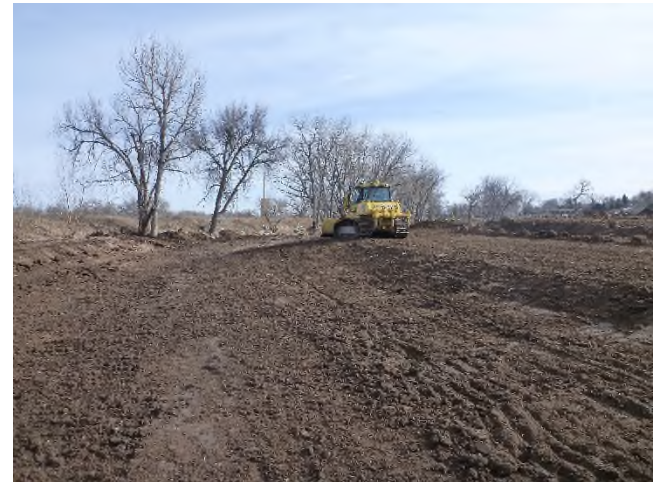
Figure 2 – Looking downstream at coarse channel grading near Sta 11+00. Final channel grading via placement of design channel bed material has not yet been completed.
