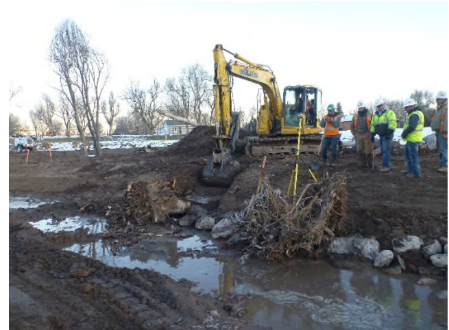
Figure 1 – Looking downstream near Sta 1+00 at rootwad installation on right bank. Final channel grading via placement of design channel bed material has not yet been completed.
