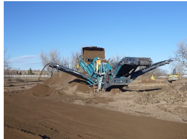
Figure 2 – Looking North across the floodplain as channel bed material is sorted via a power screen and stockpiled for later use to shape the in-channel riffles and pools.
