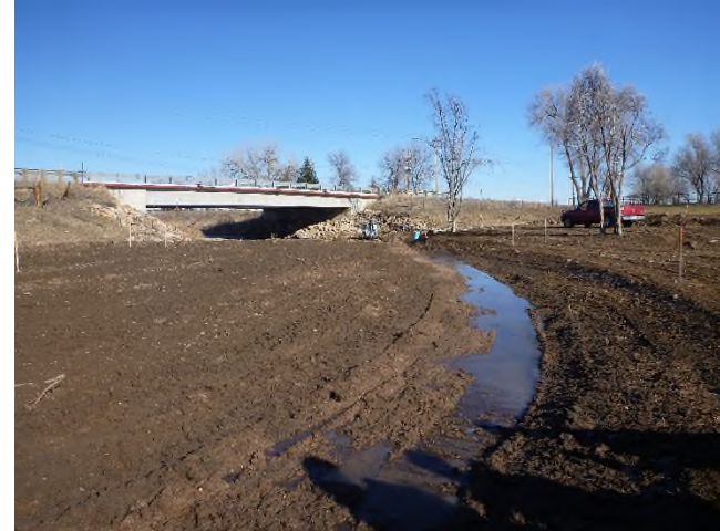
Figure 1 – Looking downstream at Sta 2+00 at coarse channel grading before low flow channel and pool are shaped. Rootwads will be installed on right bank. CR4 Bridge in the background.
