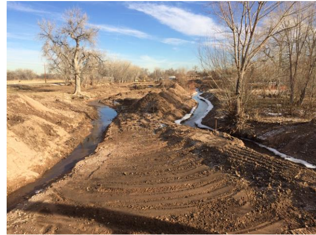
Figure 1 – Standing on Green Bridge looking east. The main channel is on the left, the diversion channel is on the right.
