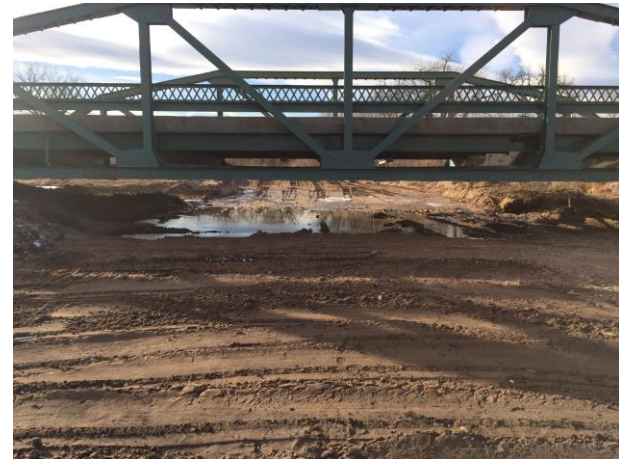
Figure 2 – Looking west at completed sediment removal under Green Bridge. Diversion channel runs to the left of this photo.
